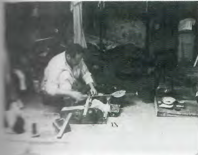
Egyptian plumber working with lead on Omar Khayyam Marriott Hotel project, Cairo (1978).
