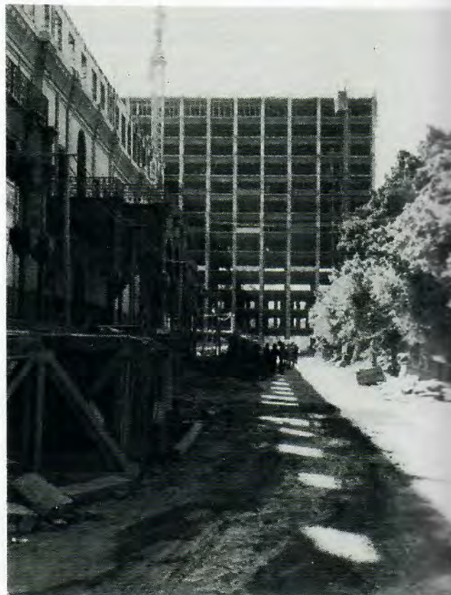
Early construction phase of the south tower, Omar Khayyam Marriott Hotel project, located in Cairo (1978).
