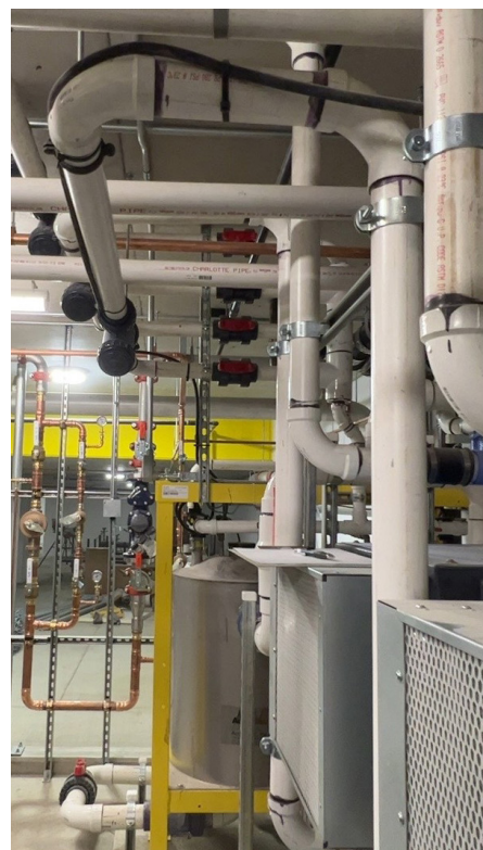
By installing AcornVac’s water-saving vacuum plumbing system in its renovation of an historic office building, Holaday-Parks earned the building recognition for environmental sustainability. The building’s AcornVac mid-level waste collection tank captures waste from upper-floor fixtures; here, it is supported by a framework (see the yellow bar).
