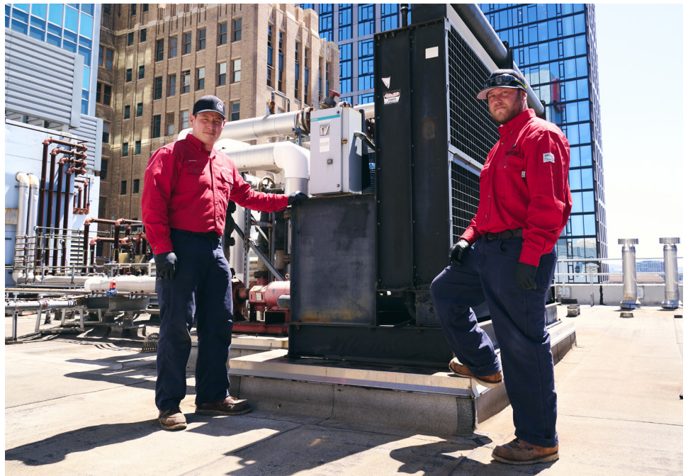
With ServiceTrade software, Western Allied Mechanical cut the time from identifying a repair in the field to sending the proposal to the client by 50 percent on average, which means service technicians in the field like Derek Yee and Stas Yudashkin can get to work sooner.
