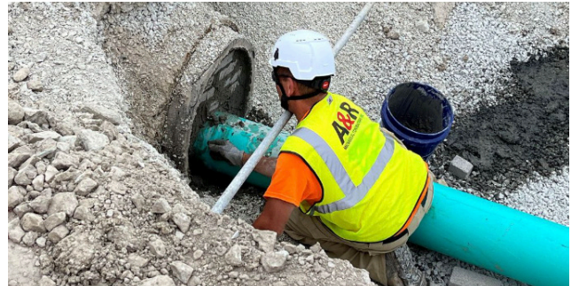
Using the Procore platform, A&R has simplified and improved scheduling and communication, so it can put the right people in the field with the right skills for the job and everyone has the information they need, resulting in a more productive team.
