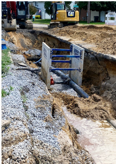
Following a spate of water main breaks, F.W. Webb fast-tracked delivery of more than 4 miles' worth of HDPE piping and accessories to replace a small city's water mains with a reliable, long-term solution.
