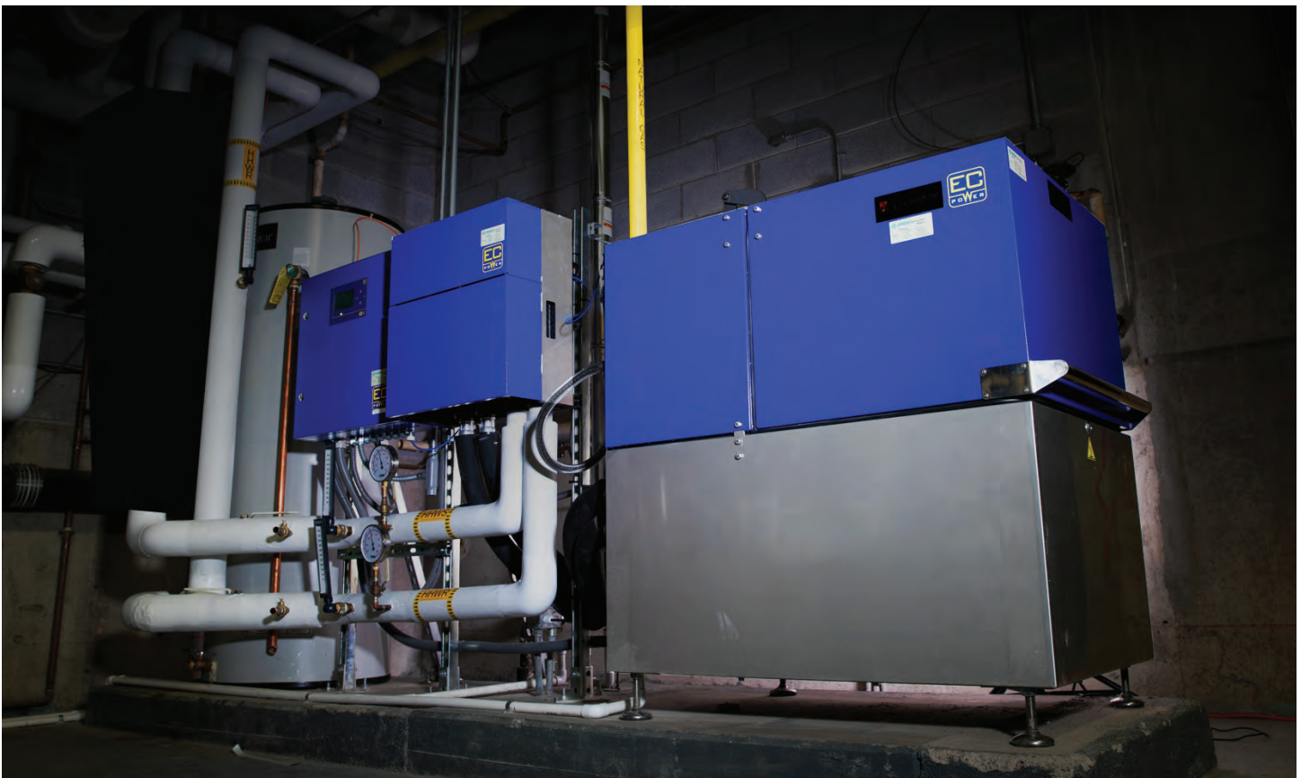
Lochinvar integrated the XRGI25 combined heat and power system with a new KNIGHT boiler system to provide hot water and space heating for Finger Lakes Community College—resulting in a cogeneration system that creates energy as it works, reducing grid dependence and lowering electrical costs.
