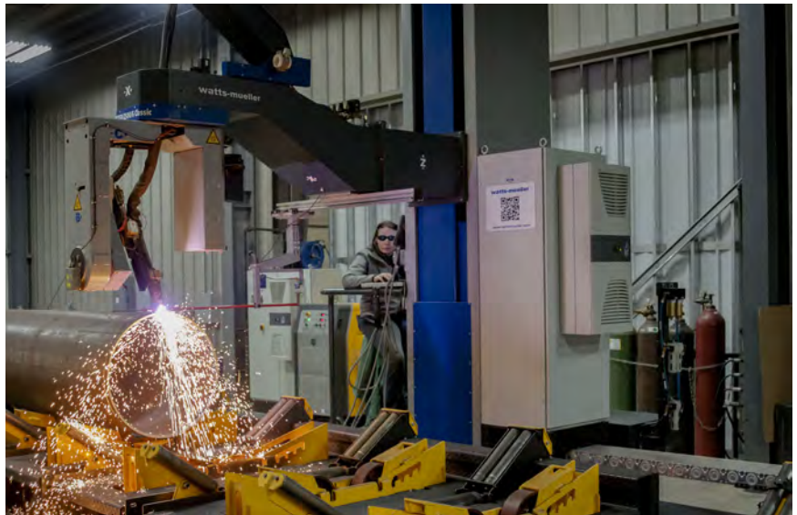
An operator rides on the cutting carriage of the Watts-Mueller WM-60, a system that allows Piping Systems to complete a job that once took seven hours in less than an hour.
