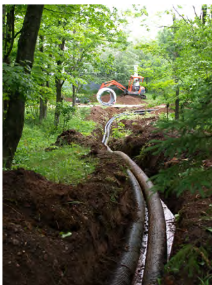
Uponor's Ecoflex preinsulated piping, proposed by McKinstry, comes in long coil lengths up to 600', so workers did not need to stop often to make connections during installation.
