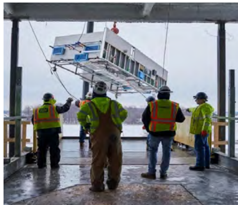
With MSUITE's FabPro software, Limbach successfully streamlined operations in a pop-up fabrication shop with multiple trades, minimizing assembly and installation time. Prefabricating units like this one ultimately cut the project time line by two months.
