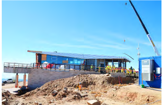
Viega certifies many of its products, including ProPress, to the stringent LBC requirements, so Olson was confident that the products they used for the Pikes Peak Summit Complex would meet the LBC standards.
