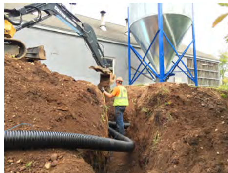
McKinstry recommended mounding the backfilled material over the new Ecoflex pipe to distribute surface water runoff and mitigate a problem that hampered the previously installed fiberglass pipe. The first winter after the installation, Wolf Ridge saved approximately $7,000 in fuel supply costs thanks to the changes suggested by McKinstry.
