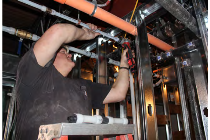
Dan Pederson, plumber with Saladino, was part of the team that quickly and easily replaced a Kansas University dorm's worn copper plumbing with 12,000' of Uponor PEX piping with ProPEX engineered polymer and lead-free brass fittings.
