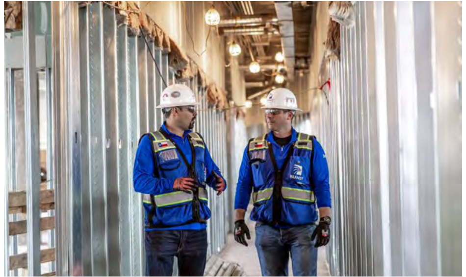
Brandt used easy-to-install HoldRite products to meet the demanding construction deadlines for a new, 12-story, two building assisted living facility in Dallas. Here, Andrew Meshell, project superintendent, and Spencer Jackson, project manager, walk through the jobsite.
