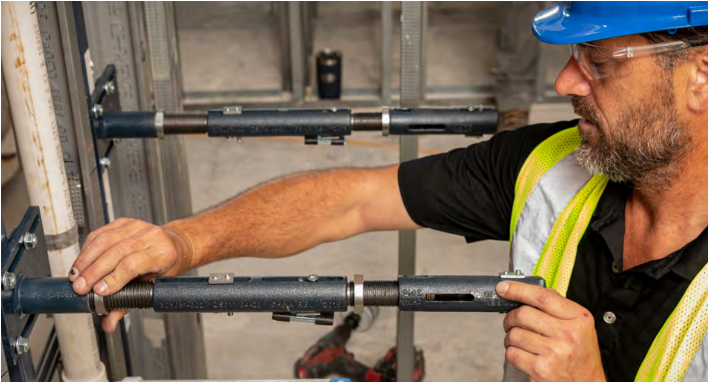
Zurn's EZ Lavatory Carrier has universal arms that can be adjusted in the field, as shown here, which simplified installation for J.M. Brennan's crew.
