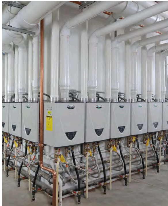
NOP came up with a unique wall-mounted installation of A. O. Smith tankless water heaters that cut down installation costs and also saved mechanical room floor space.
