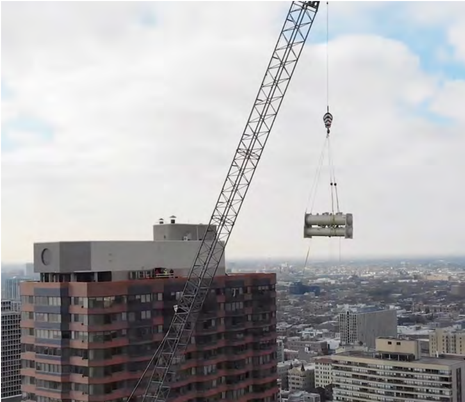
Top: Working closely with the city, Daikin erected a crane to install Brookdale Senior Living Center’s new chiller, removed the old machine, and disassembled the crane in less than 24 hours, so services to residents and neighbors continued without interruption.
