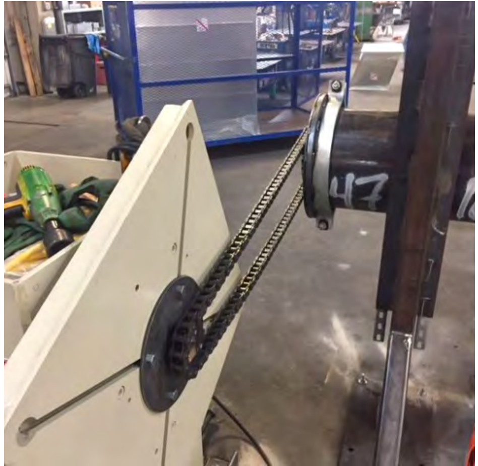
Hermanson Company designed a pipe turning system using Miller Electric's compact new welder, the XMT 350 FieldPro System, and succeeded in welding connections in much less time and more safely than hand-turning the pipe.
