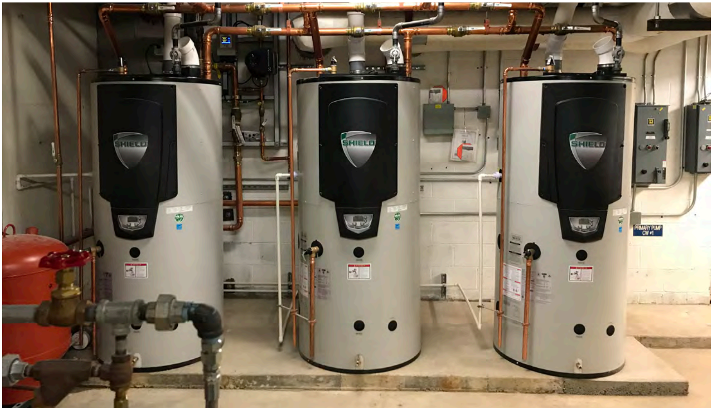
Danforth installed a new Lochinvar hot water system in a nursing home without incident and with minimal disruption, thanks in part to Ferguson's expertise in selecting the ideal replacement system.
