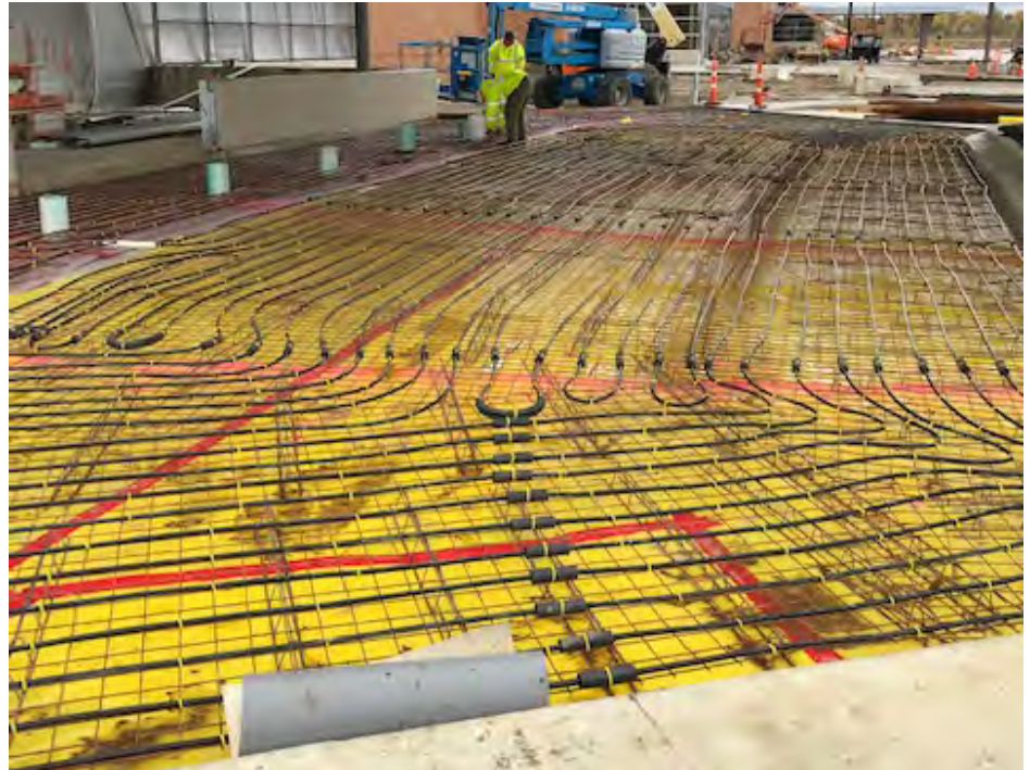
Despite having limited experience with installing snowmelt systems, crews at A&R Mechanical Contractors Inc. relied on Viega for a custom-designed system for their client in Champaign, IL, resulting in a smooth installation in time for a snowy winter season.
