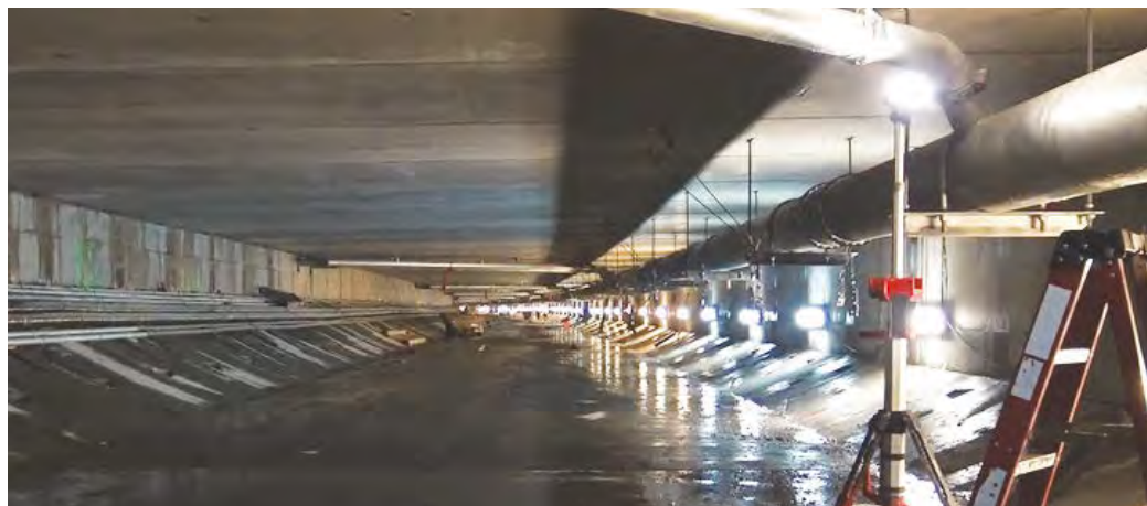
The gradual bend in the 2.5-mile long tunnel limited pipe lengths to 28 feet, which required approximately 350 pipe joints on the main line alone and made Victaulic's flexible coupling the ideal choice. Shinn Mechanical found that Milwaukee's cordless stand lights not only lit up the dark tunnel but also stood up to the harsh conditions.
