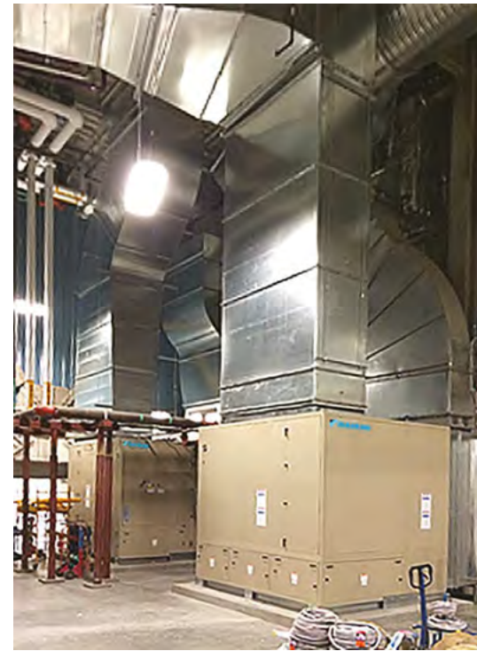
Daikin worked closely with ACCO by providing 3D CAD files of the 100-ton water-cooled Self-Contained AC units to assist with the modeling of the equipment rooms, ductwork, and piping systems, which made for a smooth installation process.
