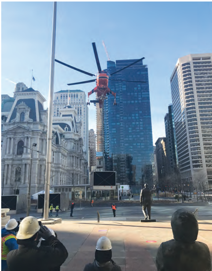
Through careful planning and coordination, Herman Goldner ensured that eight new Marley NC cooling towers were successfully placed in a downtown Philadelphia office building on schedule and in time for occupants to keep cool as temperatures rose outside.
