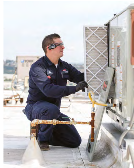
MacMiller Service Technician Neal Henry uses smart glasses equipped with a camera and software powered by XOi technology to capture his work onsite. MacMiller finds that customers pay their invoices more quickly when they can see exactly what work has been done.
