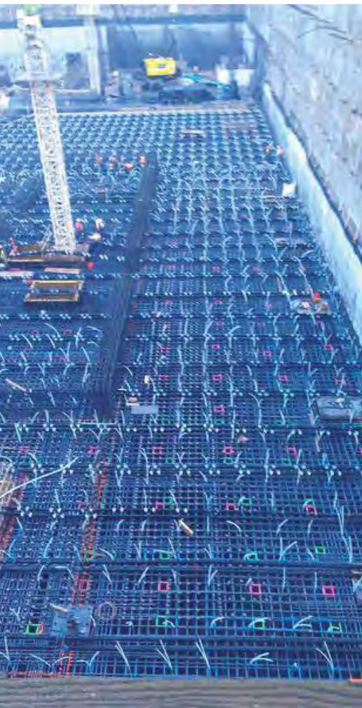
For a record-setting continuous concrete pour, Couts installed more than 20 miles of Uponor radiant tubing to create a thermal cooling system that would ensure the integrity of the concrete as it cured.
