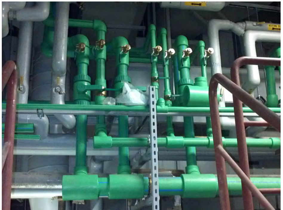
By using Aquatherm's polypropylene-random pipe systems instead of copper piping to combat the aggressive water degrading the existing pipes of the King County Jail, Auburn Mechanical saved installation time and costs.
