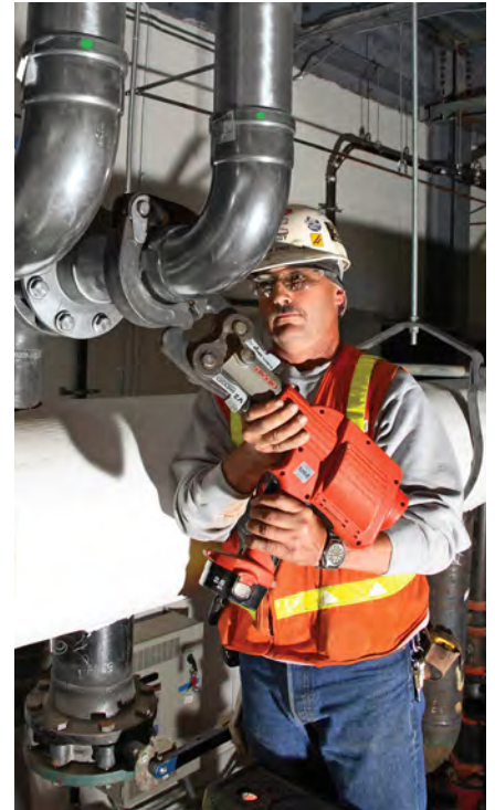
Installing Viega ProPress systems for stainless steel required about one third less time than welding would have required, enabling Hart Engineering to repipe an entire pharmaceutical manufacturing plant in 14 weeks.
