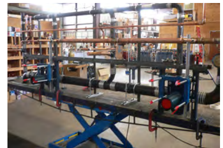
CFI Mechanical prefabricated these toilet batteries and other structures for the Smith Clinic in its shop, relying on TSI software to improve productivity and gain a competitive edge.
