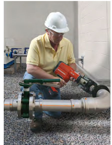
Viega ProPress systems do not require a welding permit, which was especially important when Hart Engineering replaced all of the existing piping with stainless steel for a biotechnology manufacturing client.
