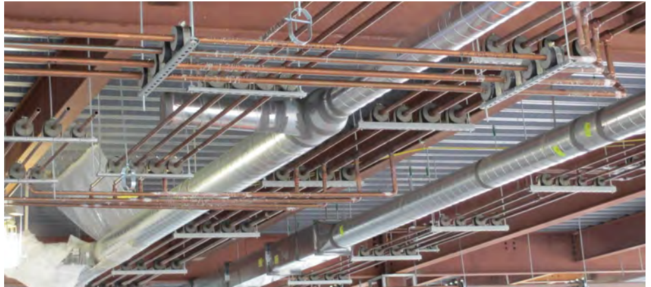
Smith & Oby is using ERICO's CADDY ROD LOCK system to install 250 active chilled beams in an office building. With the new system, instead of rotating threaded rod, workers push them into position, saving installation time.
