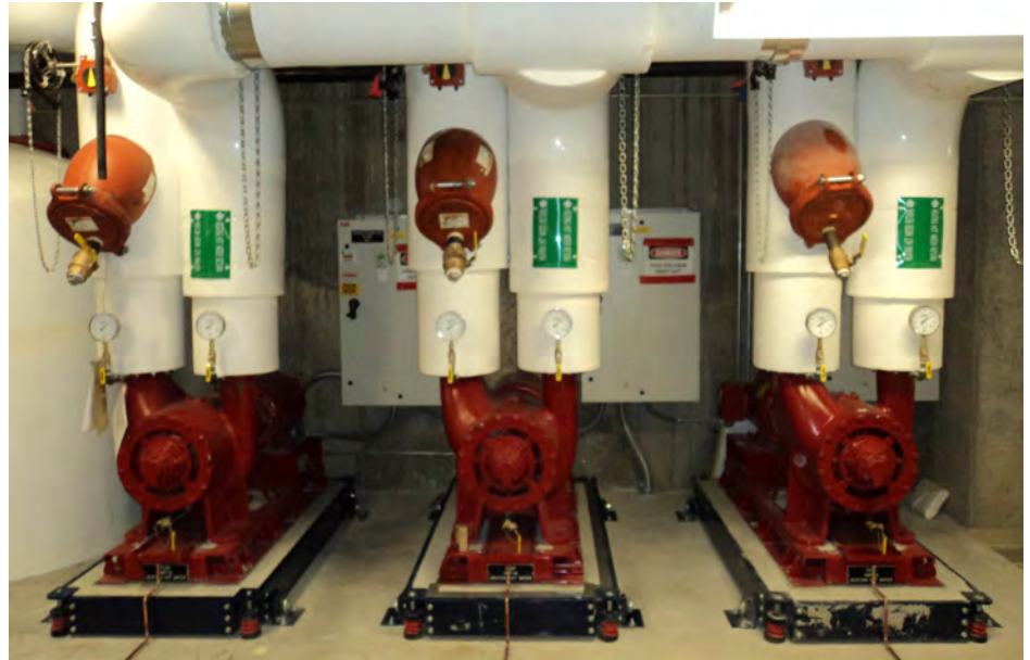
Prefabricating with grooved systems like Victaulic's keeps U.S. Engineering competitive through improved control over project schedules, faster installation, reduced labor, and increased safety.
