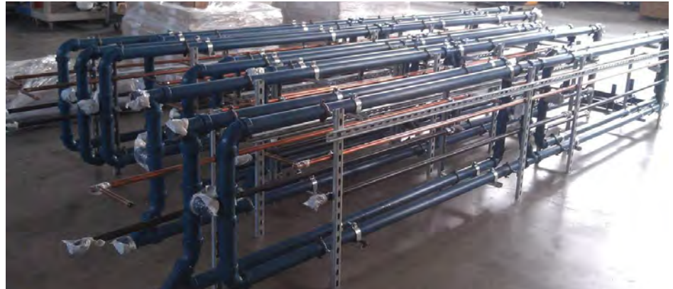
Hospitals have unique requirements, such as these pipes that pull acid away from drains. CFI Mechanical relied on TSI BIM software to coordinate and keep track of the complex and competing demands for Houston's new Smith Clinic.
