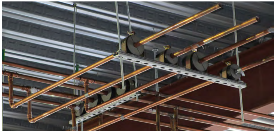
For a large office building project, Smith & Oby is prefabricating copper racks in its shop, shipping them to the jobsite, inserting ERICO's CADDY ROD LOCK into the strut, then lifting the racks in place to save labor and time.
