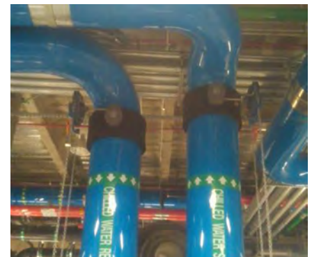
The NIBCO 14-inch LD-2000 lug-type butterfly valve with sprocket rim and chain provides remote operation on chilled water supply and return lines. Warwick specified NIBCO products for the Riverside Medical Center expansion because of NIBCO's product reliability, which has helped keep the project on time and within budget.
