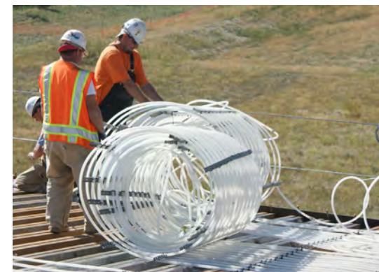
A crew at Trautman & Shreve prefabricated 42 miles of Uponor radiant tubing into mats (shown here) customized for each zone of the Research Support Facility at the National Renewable Energy Laboratory, ultimately saving time and labor costs.
