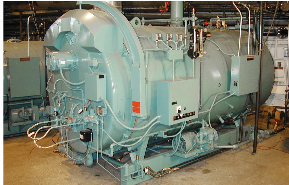
Boiler used to maintain temperature in building spaces by transferring heated fluid through piping.
