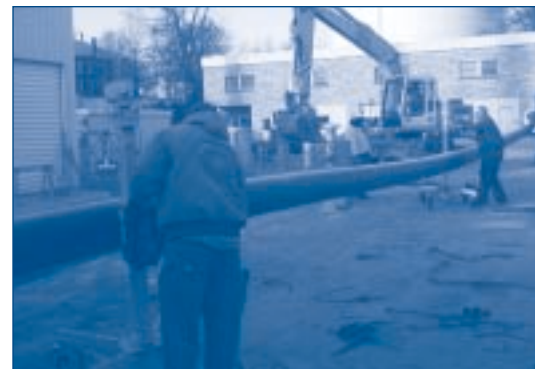
Corrigan Company employees at work on a chilled water loop renovation project at Southeast Missouri State University.
