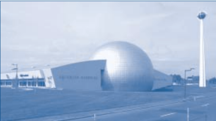
Baltimore Aircoil Company's Series 3000 Cooling Towers are part of the HVAC system at the Naismith Memorial Basketball Hall of Fame.
